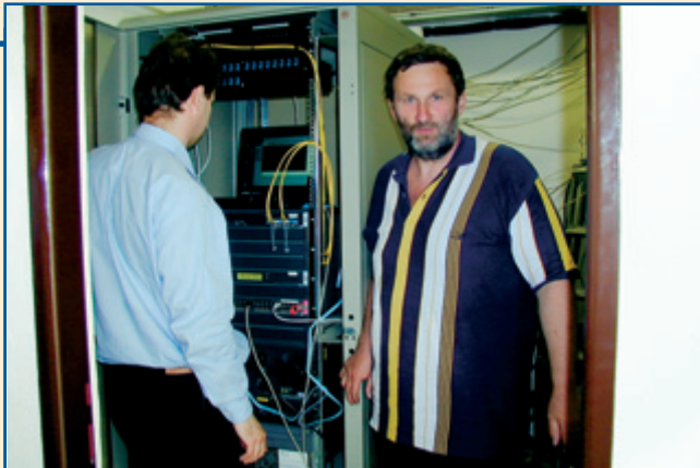
INSTALLATION OF THE SANET NETWORK NODE
