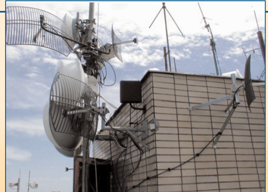
SANET RADIOCOMMUNICATION ANTENNAS ON STU BUILDING ROOF
